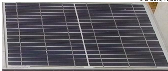
Figure 9(a): Solar panels
