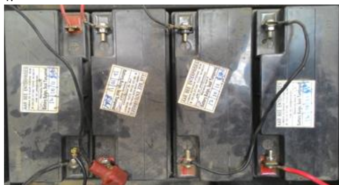
Figure 4: Batteries connected in series
